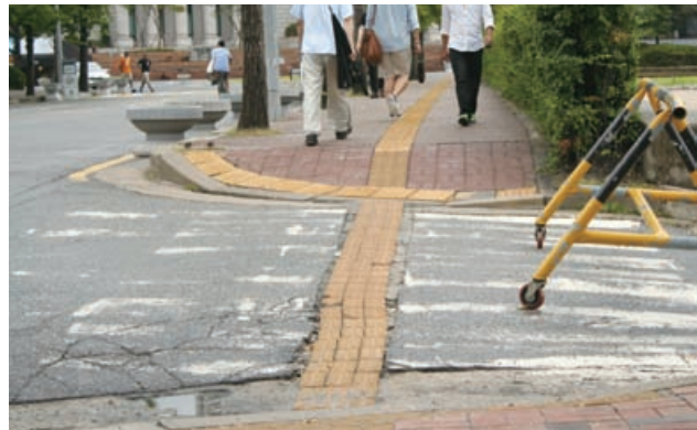
▲ Cracks on the road hinder the handicapped people from moving straight.
