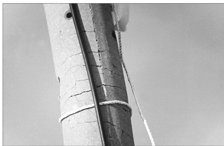
Cracks on electronic pole close to firing range are showing the serious noise problem.
