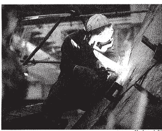
A certain laborer is working in dangerous situation without any safety device.
